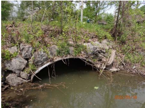
Above: Existing CSP Pipe in Poor Condition
